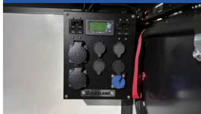
Power Supply Box (AC+DC)
